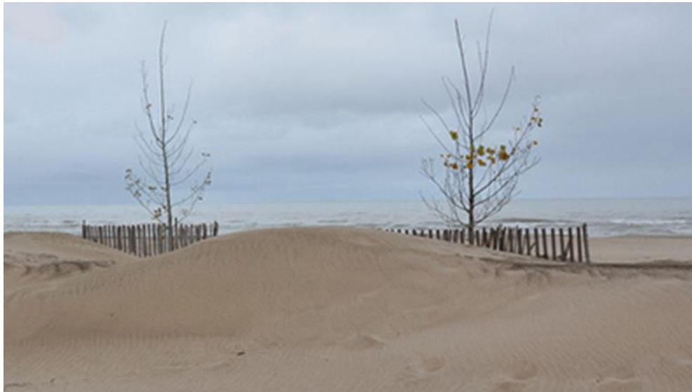
Figure 1.6 Structural sand fence installed along the coast (Source: www.flickr.com/photos/57744973@N00/8171874728 ).
